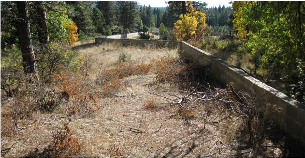
Burney Creek Floodwall
